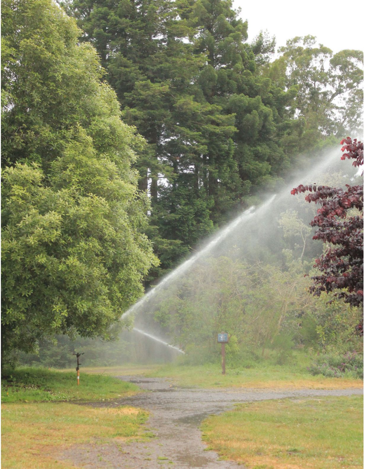
Figure 2.33 Irrigation at a park entrance, near Fulton Street and 8th Avenue.
