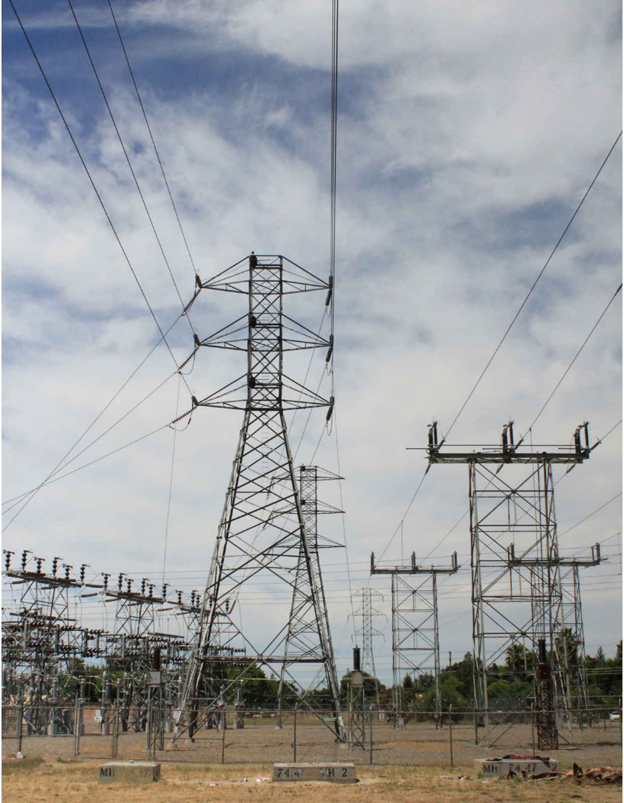
Figure 2.61 Power substation along the Hetch Hetchy Trail.
