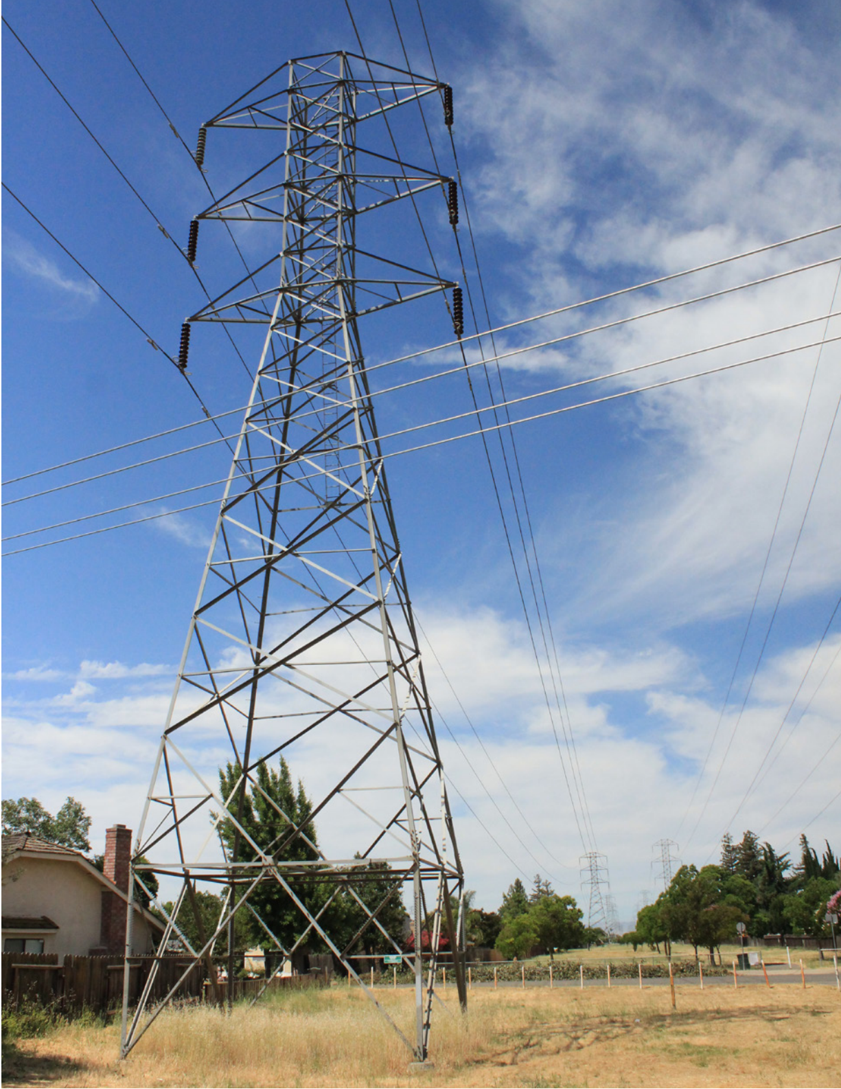
Figure 2.60 Power Pylons on the Hetch Hetchy Trail.
