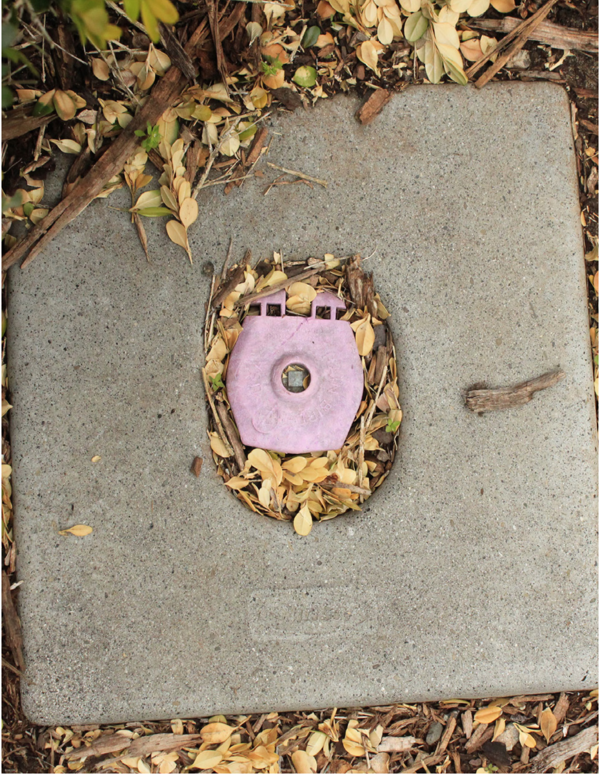
Figure 2.31 A built-in irrigation valve, to which an irrigation sprinkler would be connected.
