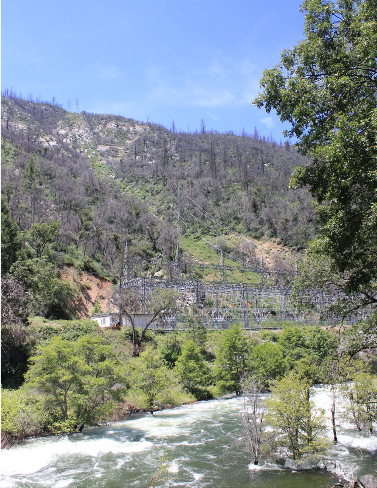
Figure 2.74 Hetch Hetchy Substation, seen on the road to Cherry Lake.
