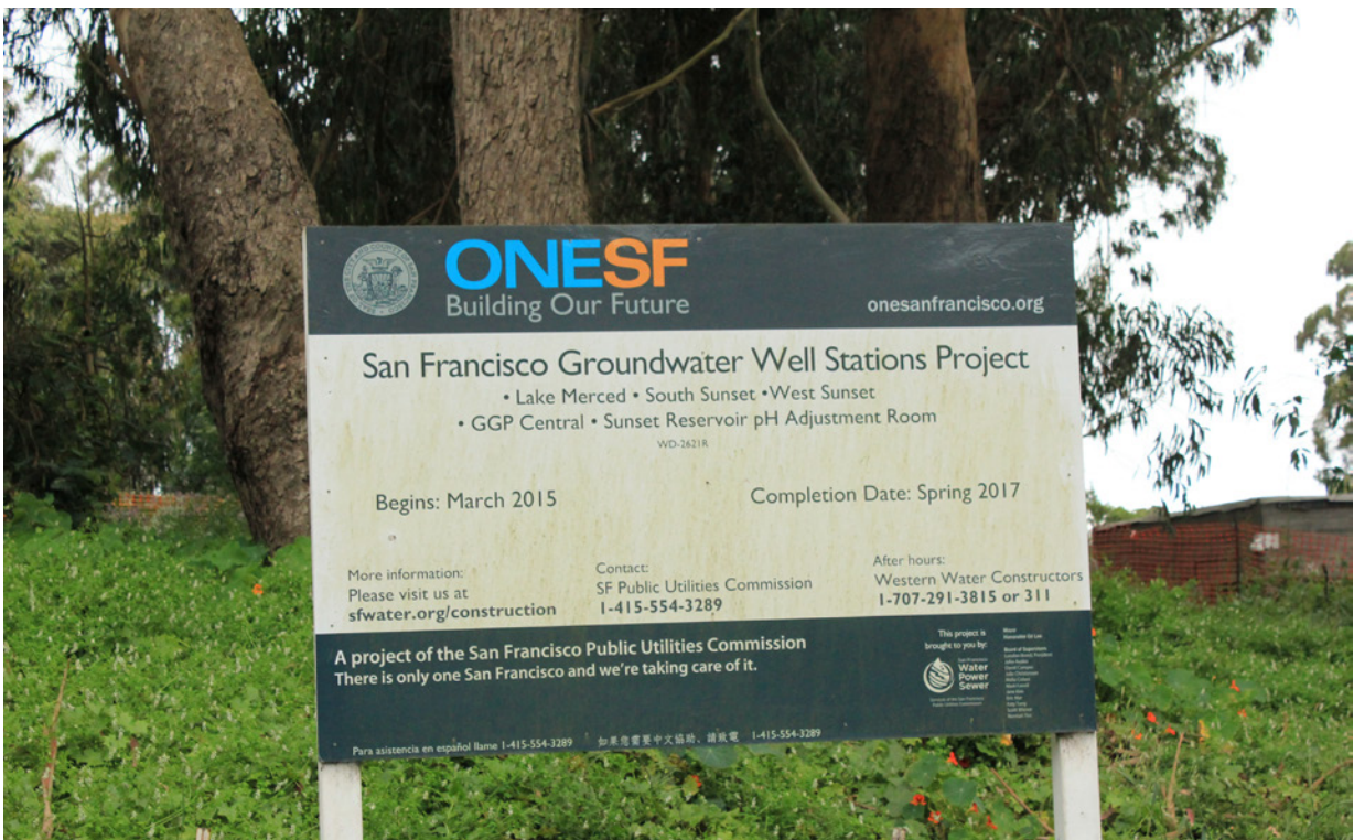
Figure 2.28 and 2.29 Water infrastructure under construction on Overlook Drive, just west of Crossover Drive.
