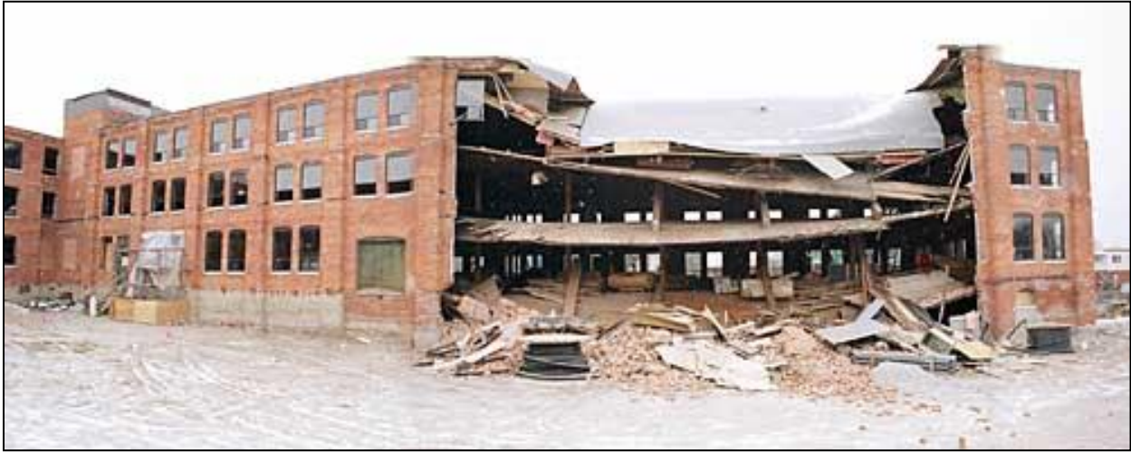
Figure 19: The Tudhope Building – Collapse During Adaptation
