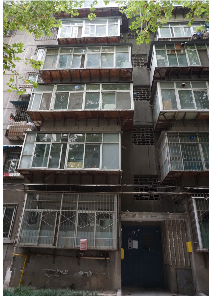
fig. 4.24 Detail of un-insulated enclosed loggia extending from the exterior wall of Socialist-era damwei housing
