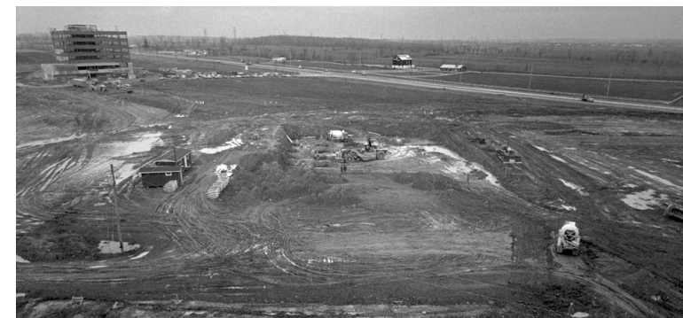
Figure 4.1 City Centre prior to construction with original City Hall in the upper left
