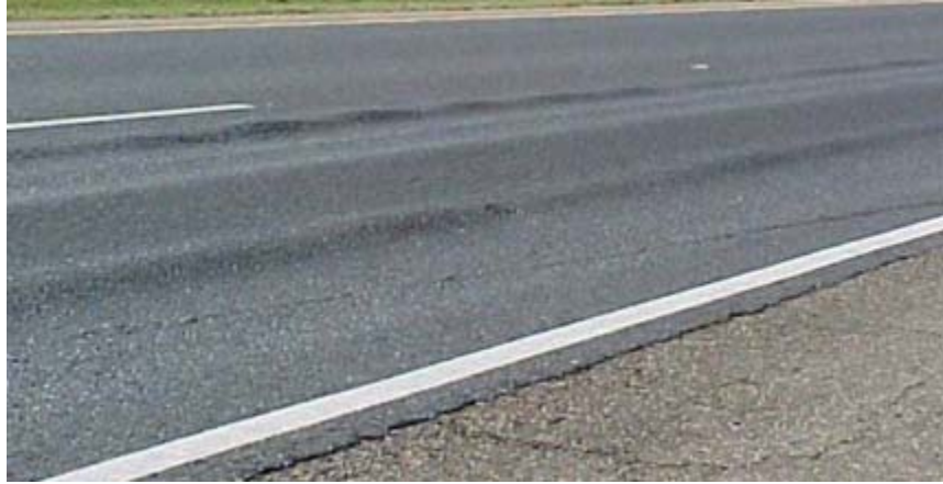
Figure 2-3 Rutting in asphalt pavement
