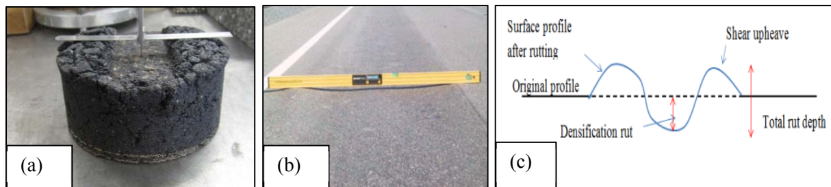
Figure 3-9 Field and laboratory measurements of HMA rutting depth: (a) total rut depth measured with a rut bar; (b) field measurement of rut depth; (c) transverse surface profile for quantifying shear upheave
