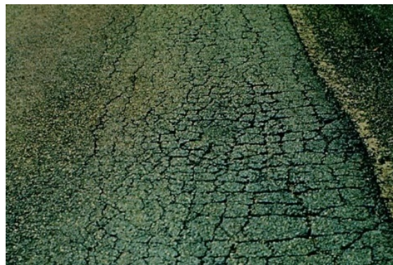
Figure 2-1 Typical fatigue cracking in asphalt pavement
