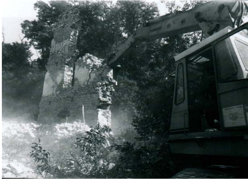
7.3 Demolition of the Parkway Mill. K-W Record Negative Collection, University of Waterloo Library.
