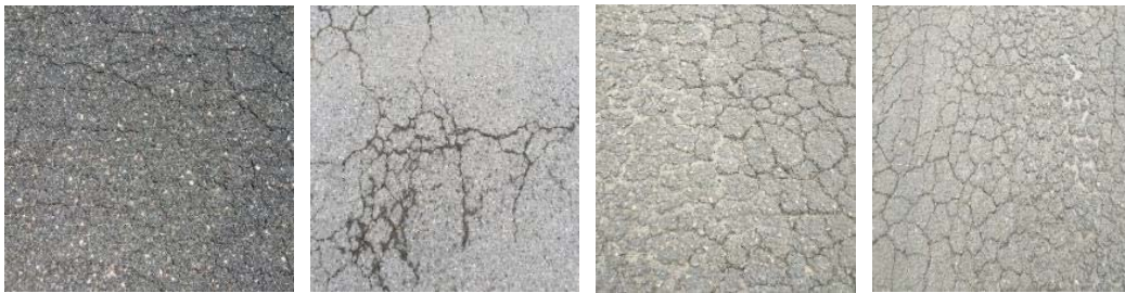
(a) Original crack images
