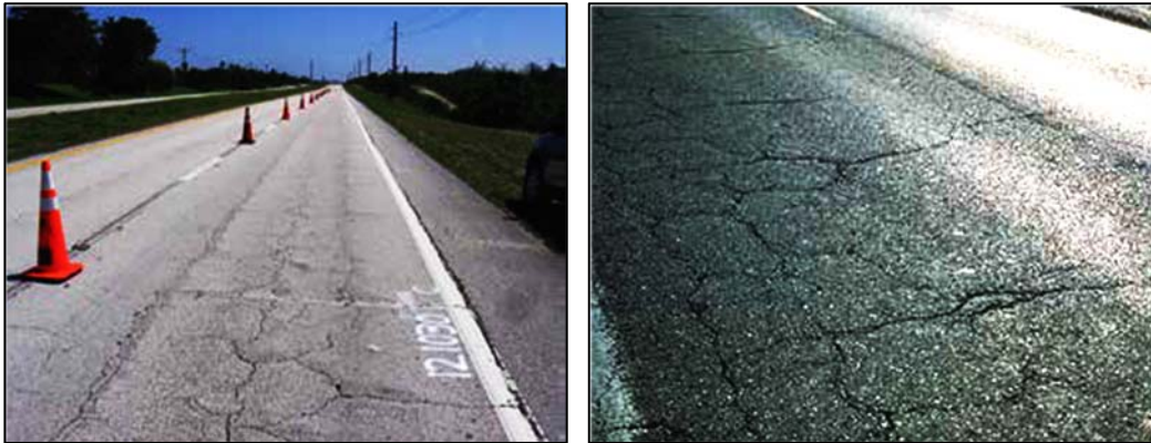
(a) Block cracking
